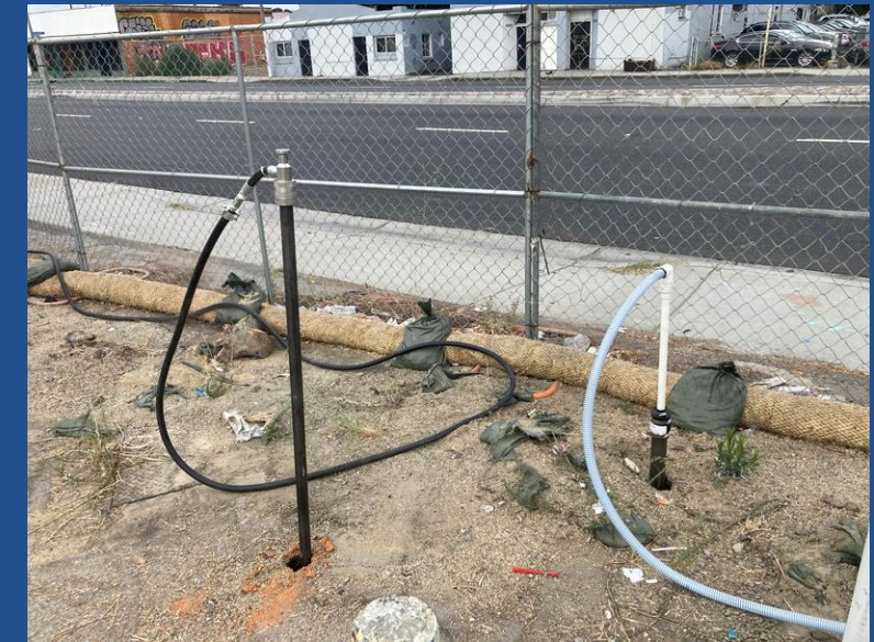
Steam location next to extraction location
